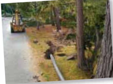
The District's sewer line replacement project uses a non-invasive "pipe bursting" technique that does not require tearing up roadways.
